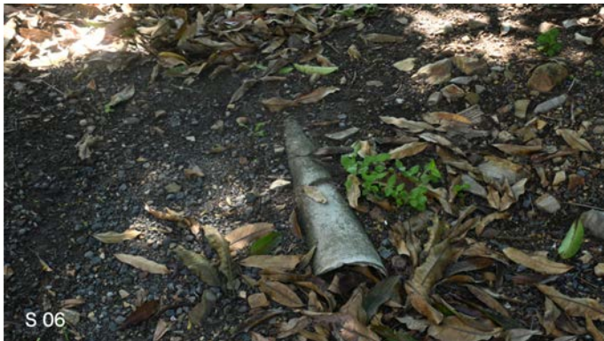
Photo 4 Exposed Pipe - Tested Positive for Asbestos
