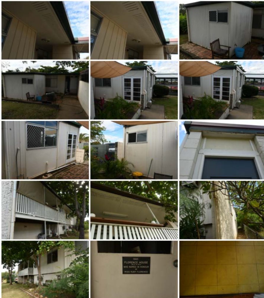
Photograph 7 Asbestos Cement Sheeting and Asbestos Tiles - Florence House
