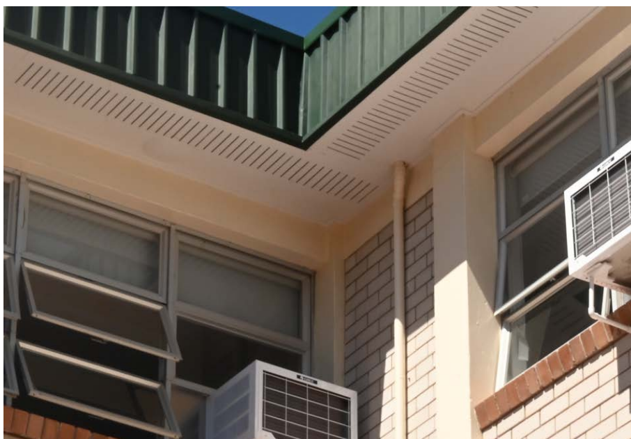
Photograph 2 Jackson House, soffits - tentatively assessed as bonded (non-friable) asbestos
