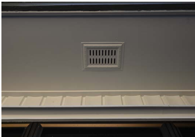
Photograph 10 Suspect material surrounding air vent of soffits
