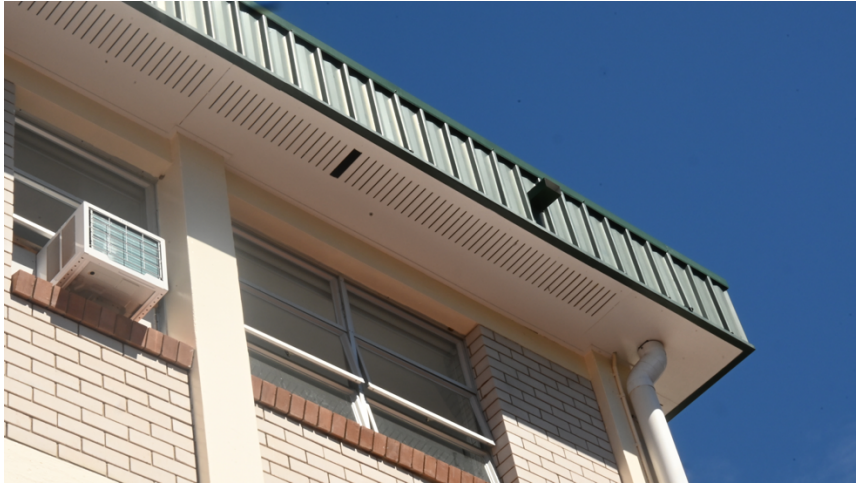
Photo 1 - Soffit of Upper Level - Presumed Asbestos Based on Testing Elsewhere
