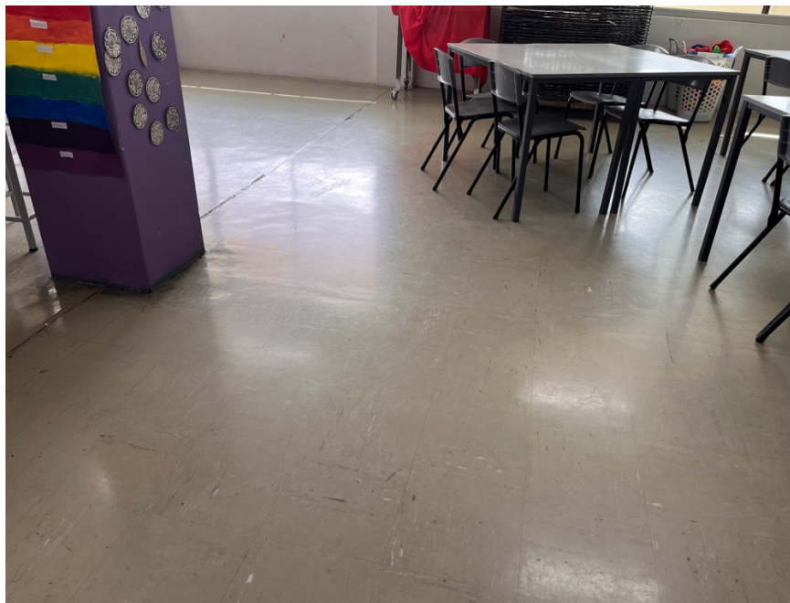
Vinyl tiles containing asbestos
