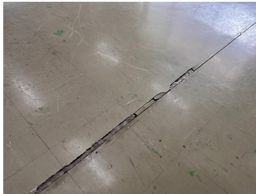
Area were cracking of tiles has occurred
