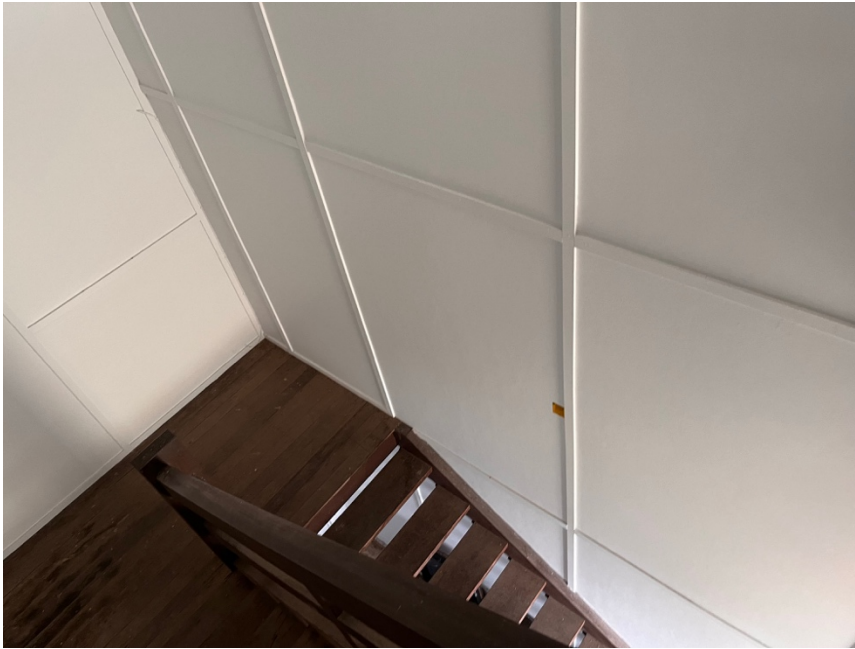
Asbestos cement wall sheeting – stairwell southern end of building
