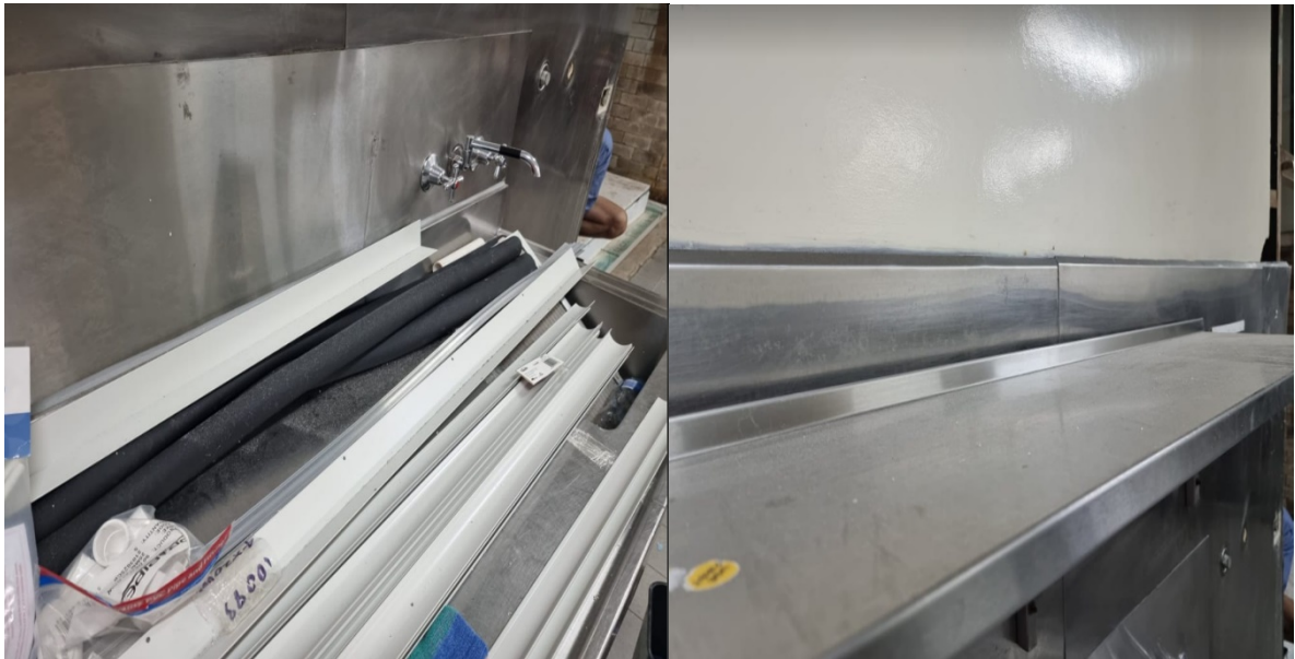
Legacy dust prior to removal
